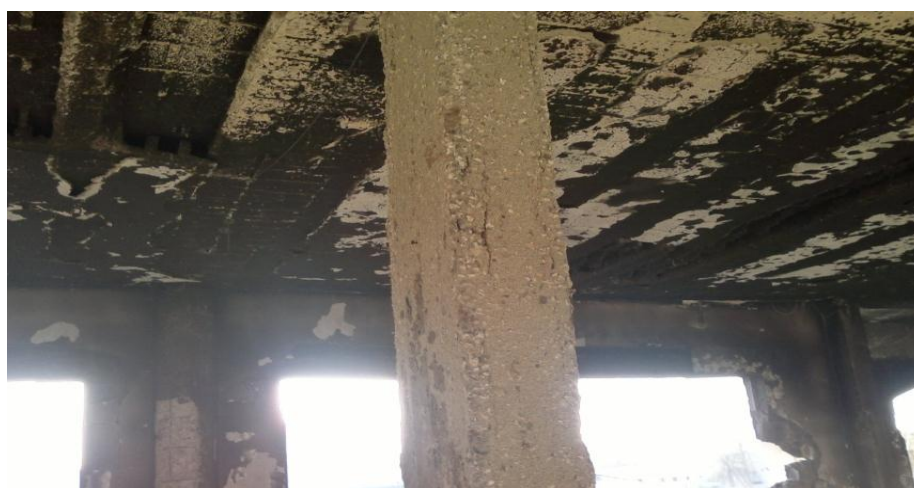
Fig. 1 A building affected by fire in Sirte
